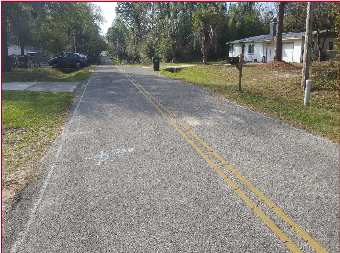
FIGURE 3B: EXISTING SITE CONDITIONG ALONG BRENT DRIVE NEAR SOIL BORING SS-4 (FACING NORTHWEST)
